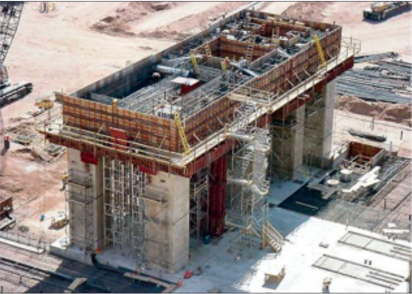
T&B products will help complete the $1 billion expansion of the Springerville, Arizona, generating station.
